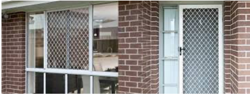
Security screens to hinged entrance doors Security screens to windows
